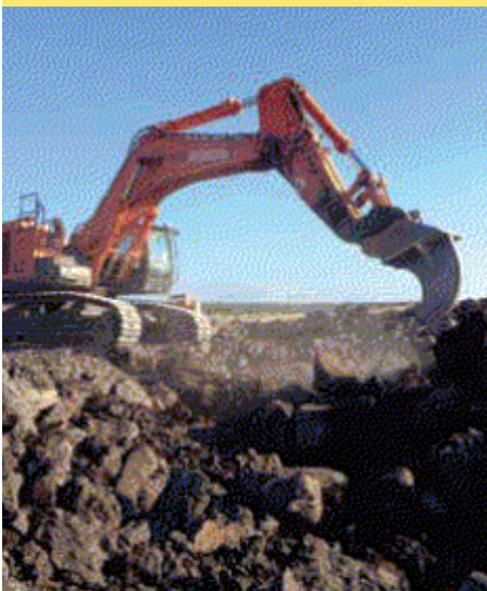
Goodfellow Bros. excavating “blue rock” at Palamanui. PHOTO COURTESY GOODFELLOW BROS. INC.
